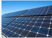
Solar Power Inverters
